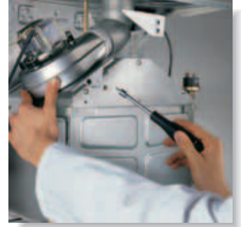
Front fan removal
